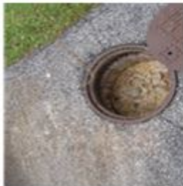
Backup due to large volumes of grease entering the sewers system.
